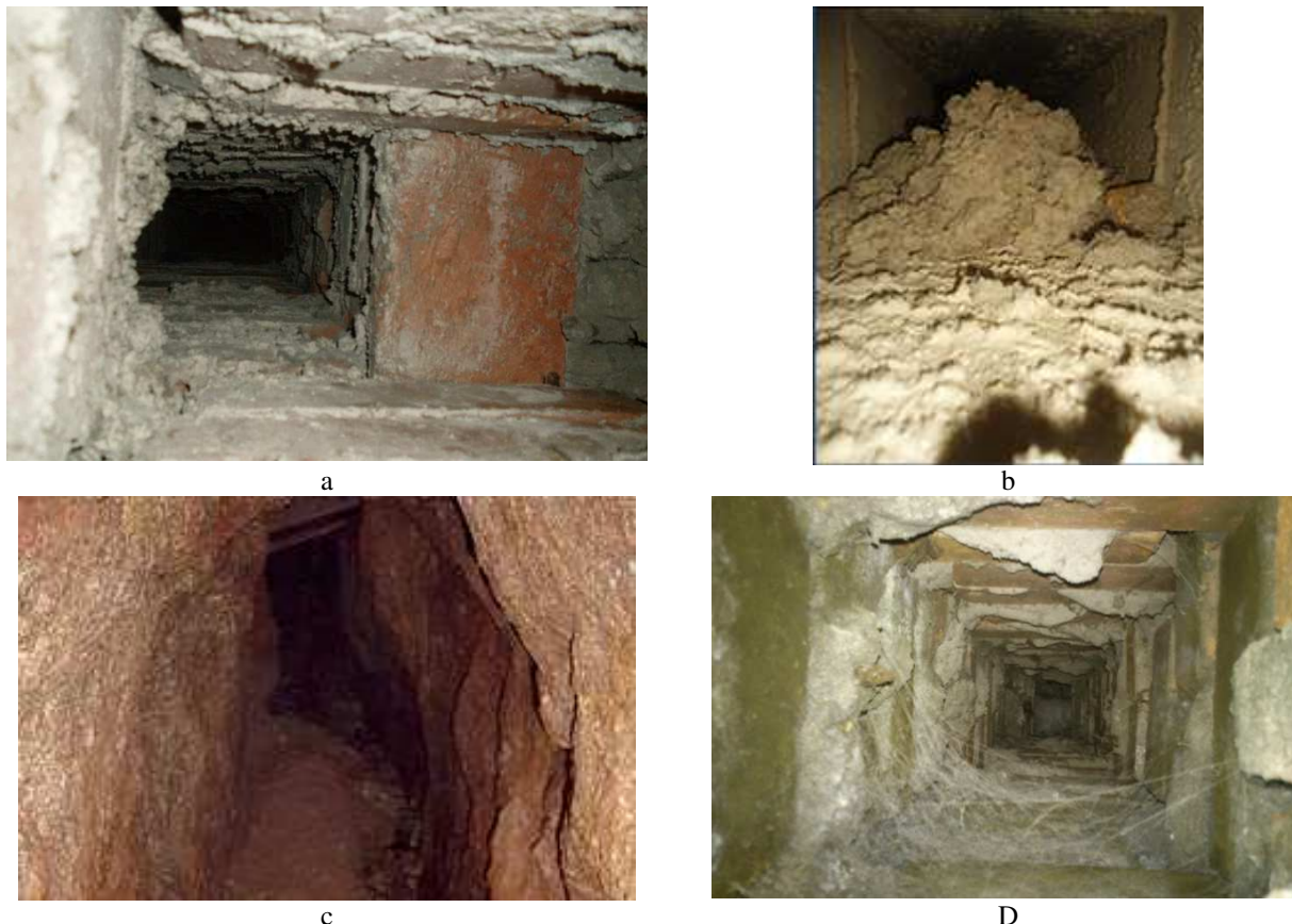
Figure 1. Possible application environments of the robot: a – standard ventilation shaft in brickwork; b – ventilation shaft with a cement barrier; c – ventilation shaft with uneven edges; d – ventilation shaft from a brick in a panel design
